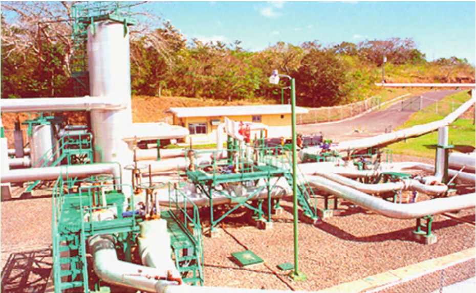
Fig. 5.3 Miravalles separator station. Photo by P. Moya [1] [WWW].
