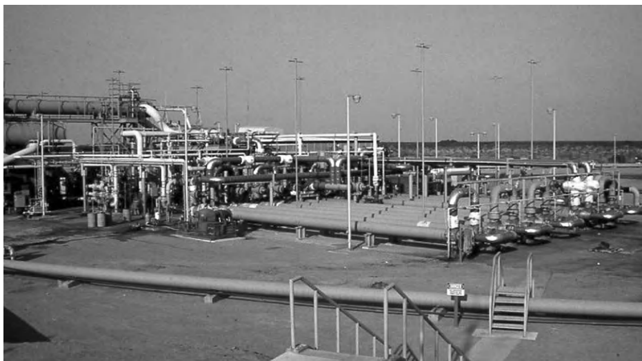
Fig. 18.2 Overview of heat exchangers, original Magmamax design. Brine-hydrocarbon heat exchangers are in center; recuperator is at upper left. June 1981, photo by author [WWW].
