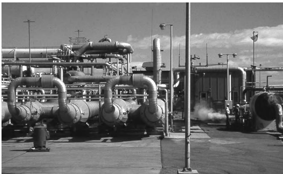
Fig. 18.11 Isobutane boiler-superheaters at redesigned plant. Note brine vertical connectors on the tube side; isobutane connectors (shell side) are seen between alternating sets of heat exchangers. October 1984, photo by author [WWW].
