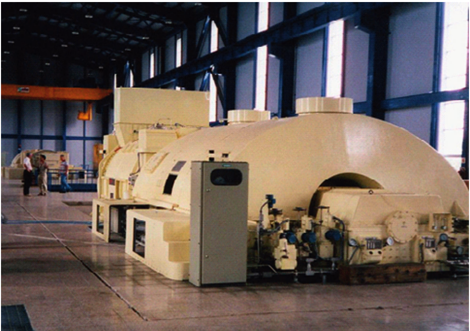
Fig. 16.8 Unit 2 turbine-generator with Unit 1 in the background; photo by author [WWW].
