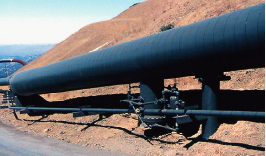
Fig. 7.7 Steam pipeline and steam trap with condensate drain line at The Geysers. Photo by author [WWW].
