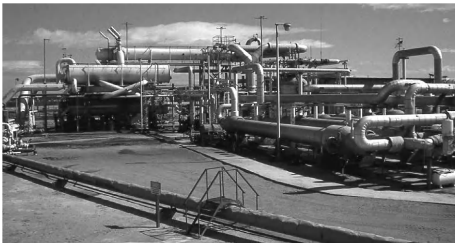
Fig. 18.10 Overview of redesigned Magmamax plant. Note new heat exchangers and the Y-connecting pipe (center) between the single exhaust of the new turbine and the recuperator. October 1984, photo by author [WWW].
