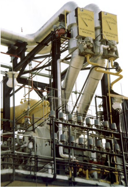
Fig. 20.14 Turbine showing dual inlet pipes, control valves, and position indicators; large horizontal pipe at left center is the exhaust pipe [WWW].
