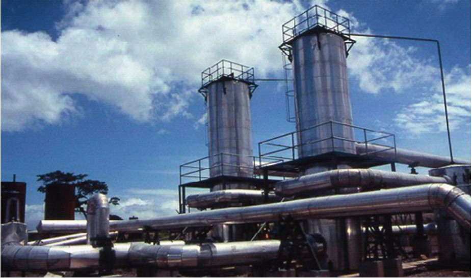
Fig. 16.7 Satellite separator station 3. Twin cyclone separators receive two-phase fluid from wells PGM-12, -20, and -21 (upper pipes at right). Steam pipes emerge from bottom of vessels (lowest pipes), and liquid is directed from the vessels into vertical surge tanks (one is visible at the far right). Photo by author [WWW].
