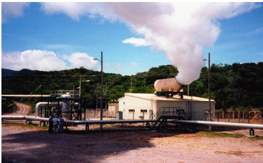
Fig. 16.9 Permanent 5 MW wellhead unit; steam is tapped from the main steam line from Satellite 1, passes through a moisture remover (left) on the way to the turbine. Exhaust steam is discharged to the atmosphere through a roof-mounted silencer. Photo by author [WWW].
