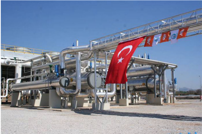
Fig. 21.15 Heat exchangers at Salavatlı Dora II plant; Level 1 is at left, Level 2 is at right [19, 20] [WWW].
