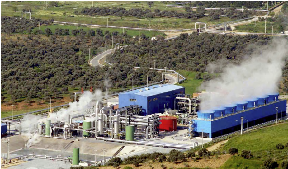
Fig. 21.22 Germencik double-flash power plant, Google Earth, image 21329604, by E. Atilir [WWW].
