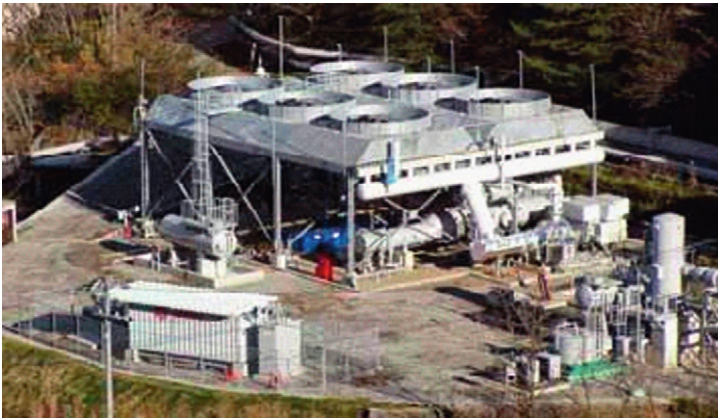
Fig. 14.12 Hatchobaru 2 MW binary unit. Photo courtesy of Ormat [17] [WWW].
