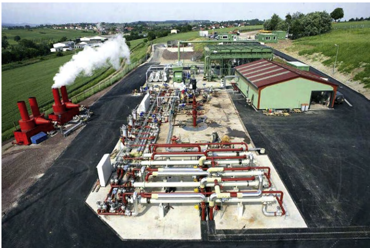
Figure 22.28 Soultz 1.5 MW pilot power plant [35] [WWW].
