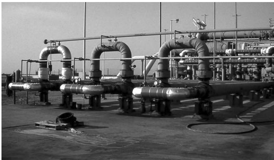
Fig. 18.3 Isobutane liquid heaters. Note vertical brine crossover pipes (shell side) and horizontal end-connectors carrying isobutane (tube side) from one heater to the next. June 1981, photo by author [WWW].
