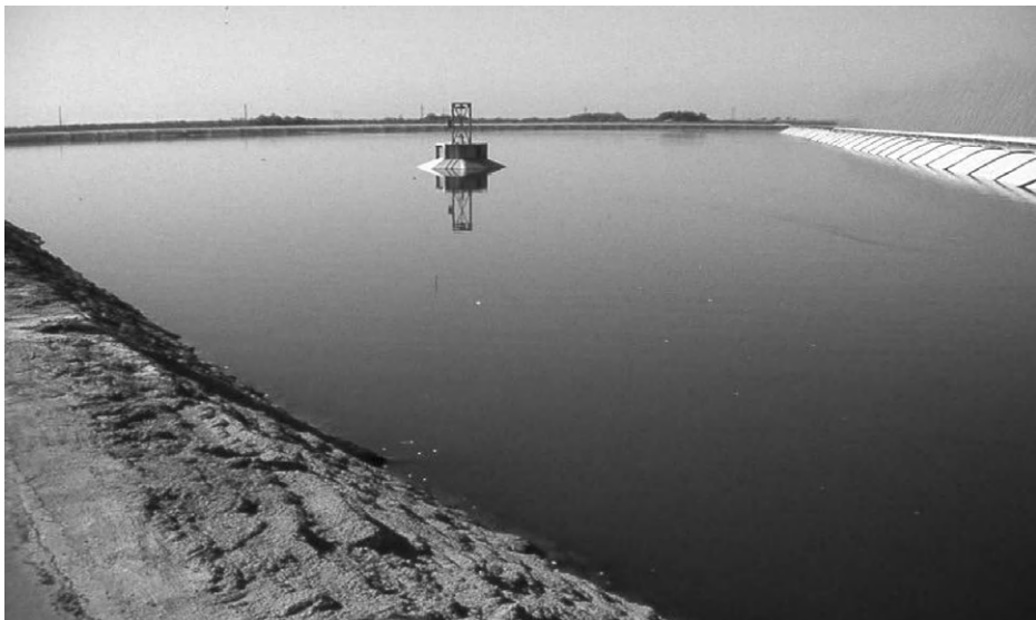
Fig. 18.8 Deep holding pond for cooling water with pump island. Note spray facility at right; cooled water drains by gravity to the holding pond. October 1980, photo by author [WWW].
