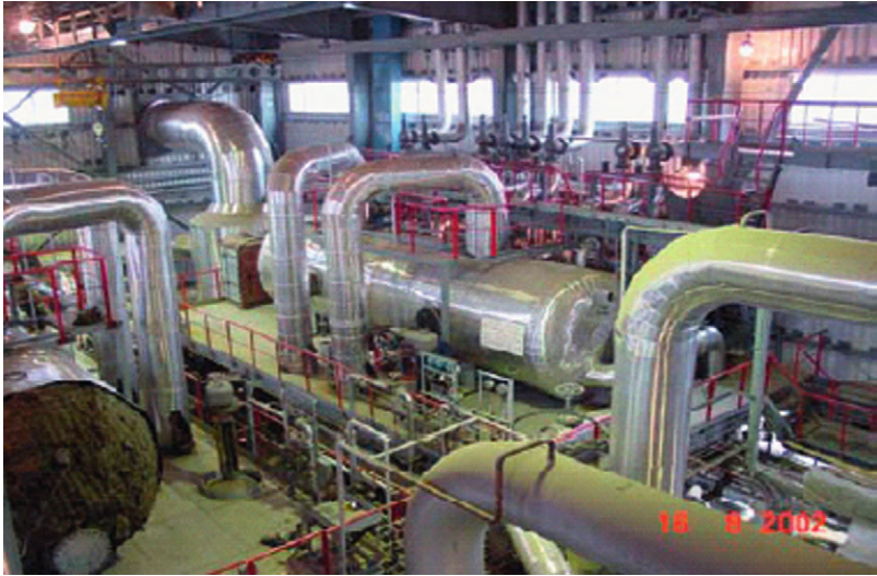
Fig. 15.10 Interior of the separator building of the Mutnovsky power plant, showing the main separators. Photo from Povarov, et al [8] [WWW].
