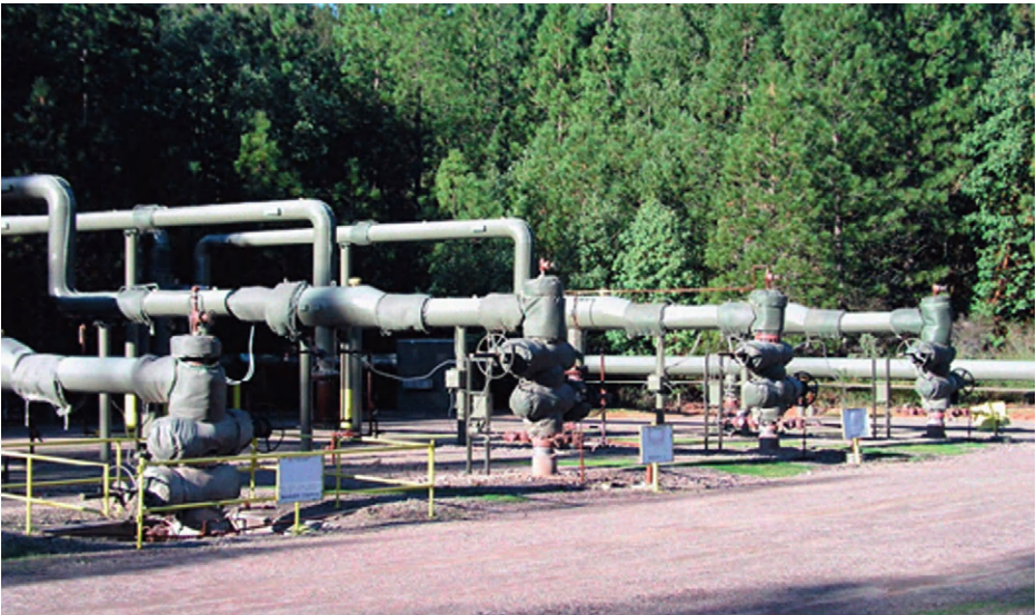
Fig. 7.6 Wellhead pipelines at The Geysers. Note axial separators to remove particulate matter. Several wells are sited on a single drilling pad to reduce the amount of land needed for well pads. The wells are drilled directionally to intercept a large reservoir volume. Photo courtesy of Calpine Corporation [17] [WWW].
