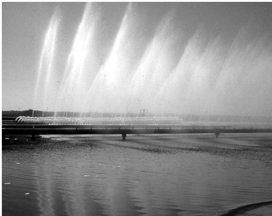
Fig. 18.7 Cooling water spray pond. October 1980, photo by author [WWW].
