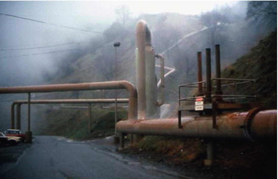
Fig. 7.8 Emergency steam relief valves at The Geysers. Photo by author [WWW].
