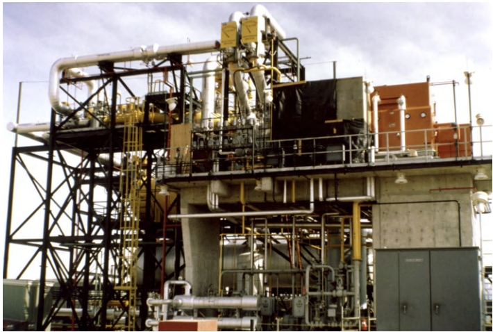
Fig. 20.13 Turbine-generator on elevated pedestal [WWW].
