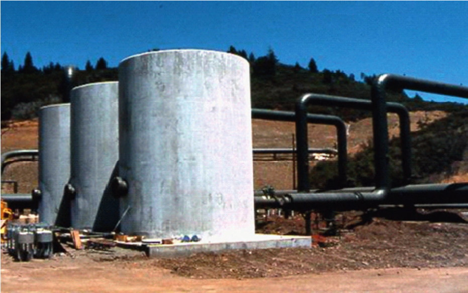
Fig. 7.9 Rock mufflers for emergency steam stacking at The Geysers. Photo by author [WWW].
