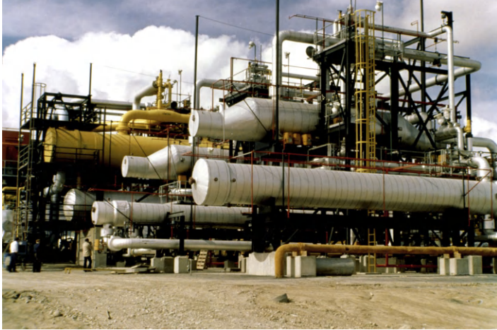
Fig. 20.11 Heat exchangers. LTH is at lower right, LPE is at upper right, HPH is at lower center, HPE is above the HPH. The condenser is the large horizontal vessel at the upper left rear [WWW].
