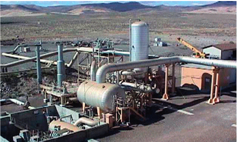
Fig. 6.5 Separator-flasher arrangement at the 17 MW Beowawe double-flash plant, Nevada, U.S.; photo by author. Two 2-phase pipelines enter from left rear; the vertical vessel is the cyclone separator and the large horizontal vessel is the flasher. The smaller horizontal vessel in the cellar is the hot water holding tank from which the waste fluid is pumped to the injection wells [WWW].
