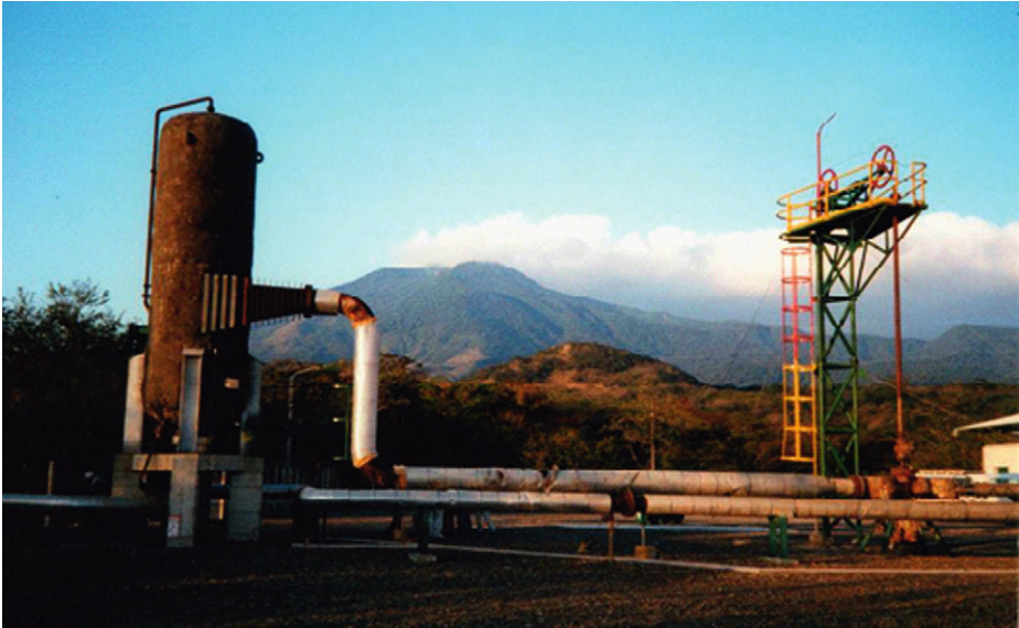
Fig. 16.13 Acid neutralization system at well PGM-19. The tower supports the lubricator and pulley assembly for the chrome-nickel capillary tubing. The control room is at the right and the cyclone separator is at the left. Photo by author [WWW].
