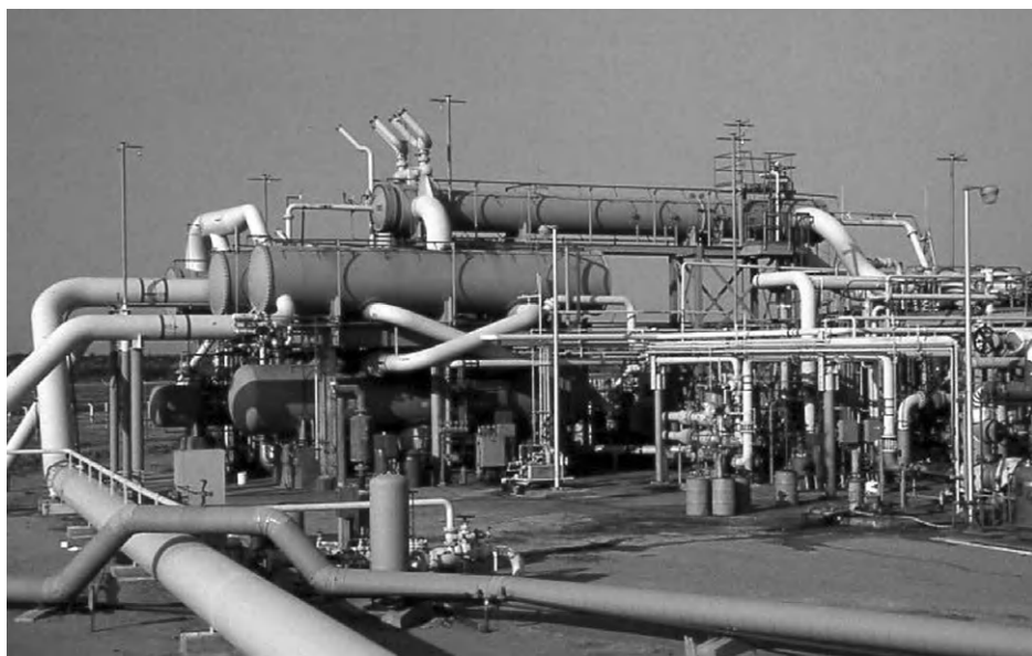
Fig. 18.4 Condensers and recuperator (upper vessel) at original plant. The two condensers on the near side are for the main isobutane cycle; the third one behind them served the propane cycle. June 1981, photo by author [WWW].
