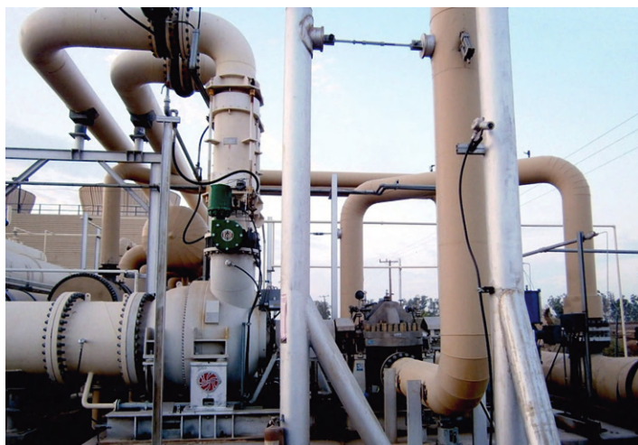
Fig. 17.9 Turbine (center left) — injection pump (center right) unit at Gould I bottoming plant south of Heber 1 double-flash plant. Photo courtesy of Ormat.
