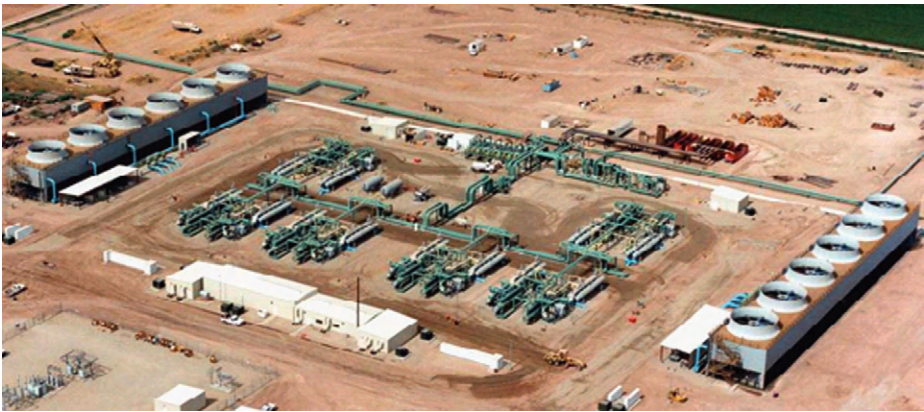
Fig. 17.6 SIGC Heber binary plant showing six clusters of ITLUs. Brine reinjection pumps are located in the upper center of the photo. The photograph in Fig. 17.5 was taken from the top of the left (southern) cooling tower. Photo courtesy of Ormat, Inc. [WWW].
